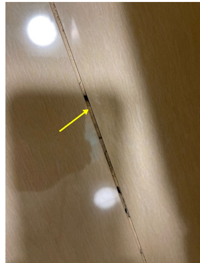
Missing and cracked grout in areas. Recommend re-grouting the floor.
