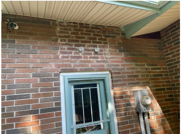
Previously repaired brick mortar. The repairs are noticeable, and not very aesthetically pleasing. Amateurish workmanship. Other than appearance the repair is acceptable.
