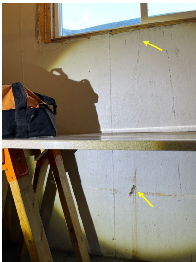
There is a crack in the foundation below the basement window. Looking at the lower part of the picture, we can see staining indicating that this crack has leaked before. Recommend crack injection to repair a crack in avoid future leaks.
