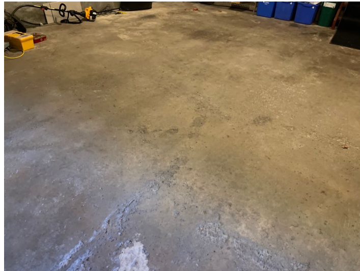
There are some common cracks in some spalling concrete in the garage
