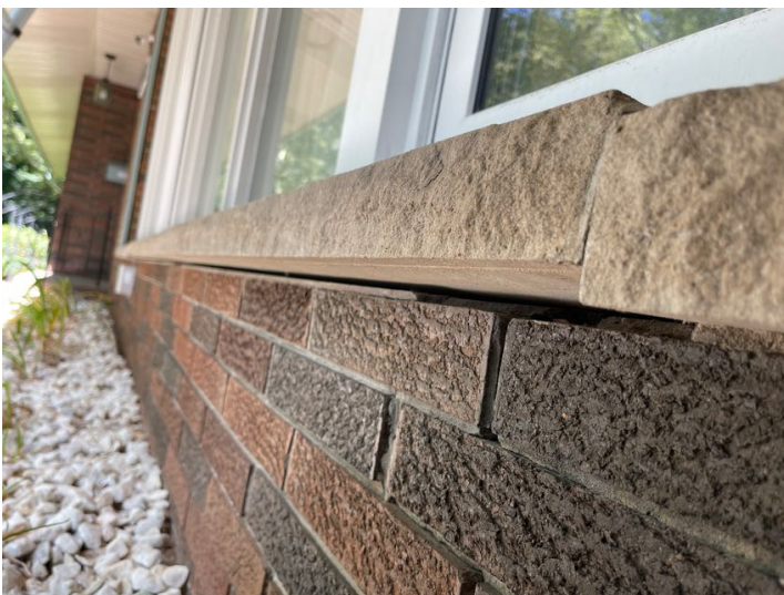
The windowsills at the front of the home are slanted towards the windows. This encourages water to flow behind the brickwork and may cause damage to the wood framing behind. Recommend removal and reinstallation of the windowsills at the front living room windows.
