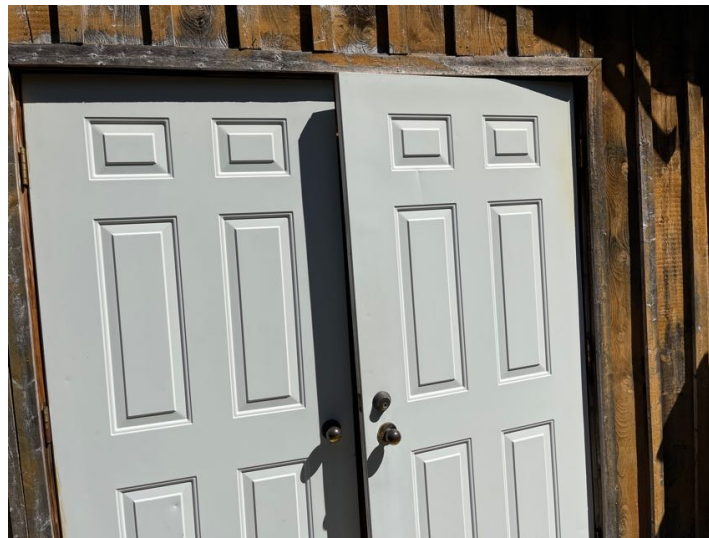
The door hinges are loose and the door does not close properly or easily. Recommend repair.
