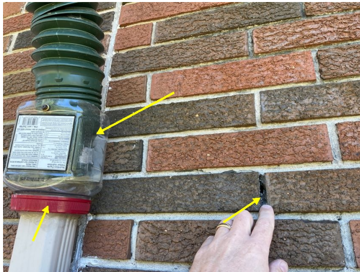
Any openings in the brick work should be re-mortared.
