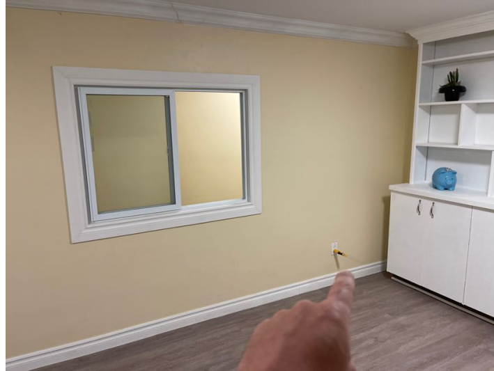
This electrical outlet is wired in reverse. Recommend electrician repair.
