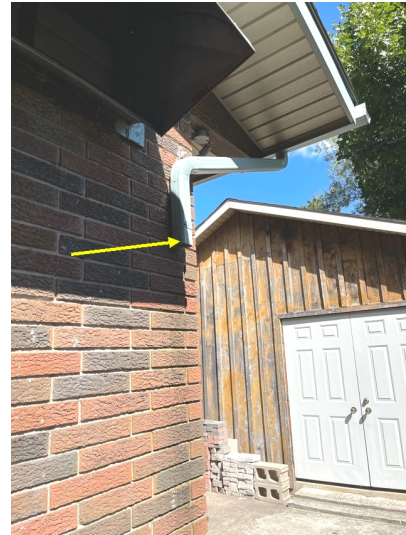
Rear right of the home. Recommend extending this downspout so that there is not water dumping it next to the foundation.
