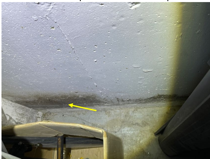
Possible organic growth on this wall, right side of the home, right of the laundry room window labelled D. Recommend cleaning with one part bleach to three parts water.
