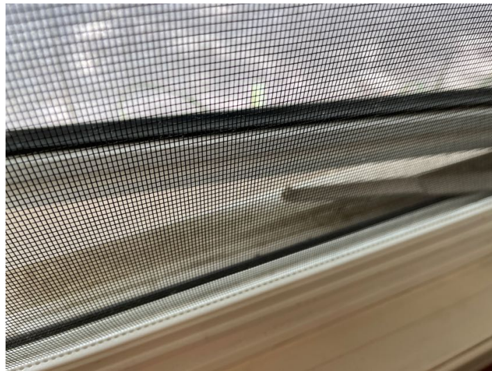
Crank arm disconnected on one of the windows in the front living room.
