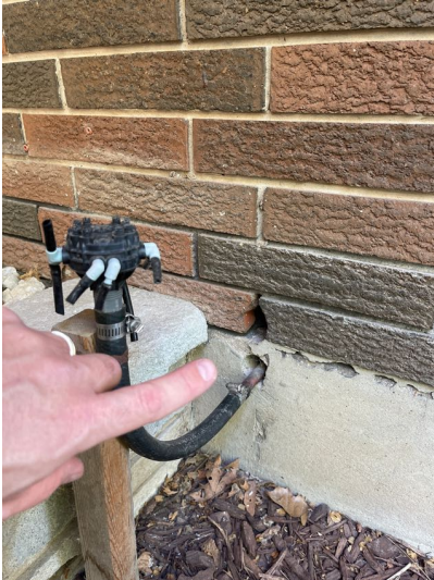
There are voids in the foundation in the brick work at the front of the home, where the pool building meets the main house. Recommend sealing these areas up to keep moisture and pests out of the home.
