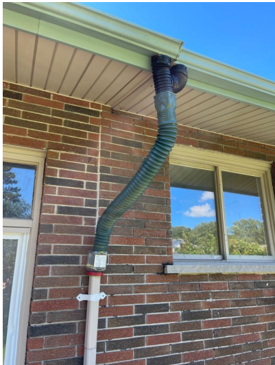
This is an unreliable connection. These accordion style extenders, crack, and break with sunlight. This gutter is also draining into an underground connection. Recommend having a proper downspout installed and discharged out on to the grass.
