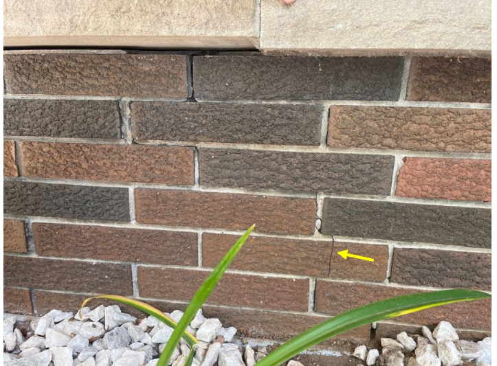
There is a crack in the brick, as well as several bricks with missing mortar in this location at the front of the home underneath the front living room windows. Recommend sealing this and re-mortering where needed.
