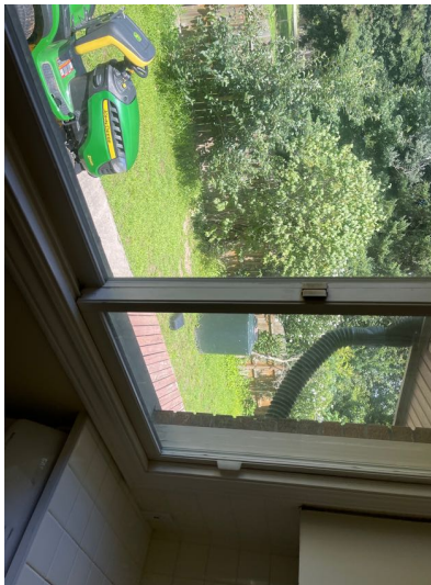
Missing screen on main level laundry room
