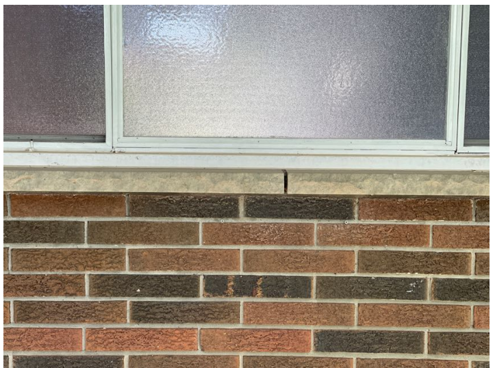
Missing mortar between two windowsills at the front of the home. Pool room. Recommend repair to avoid water infiltration behind the brick work. The other window has martyr however, it is deteriorated and needs to be replaced as well.
