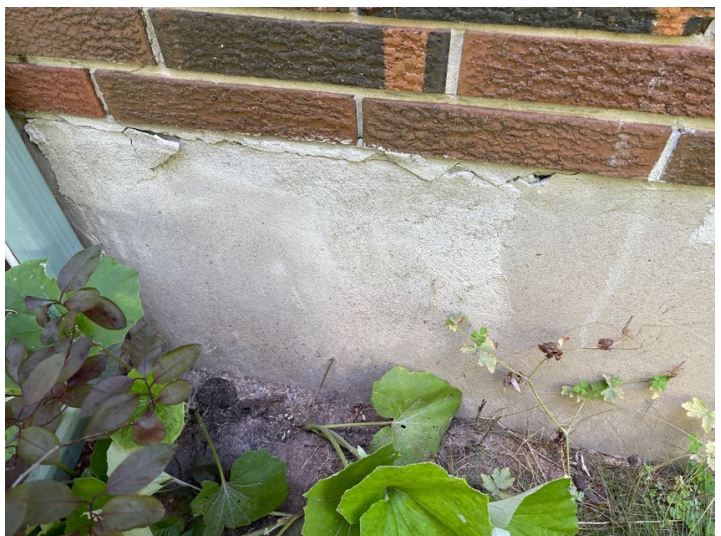
There is some damaged parging. This picture is on the left side of the home.
