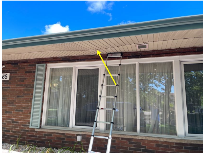
The soffit material has come loose in the section recommend reattaching soffit.
