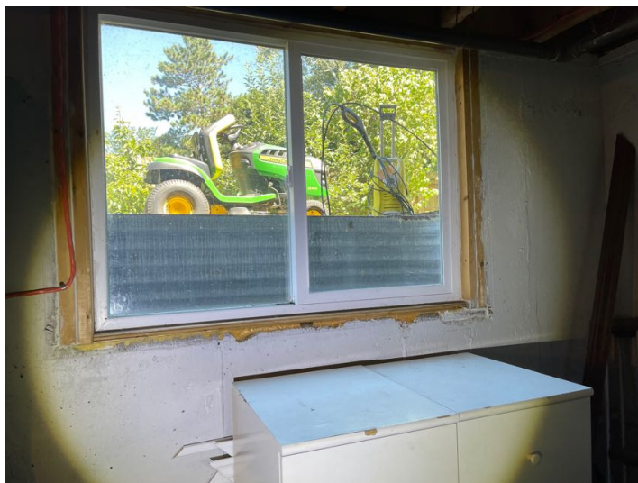
This basement window located to the right of the dryer, has a crack diagonally on the right side of the window. This is an extremely fine crack and not likely to leak, but not impossible to leak. You may wish to have this crack injected, depending if you are comfortable with the risk of leaving it or not. See picture D for close-up
