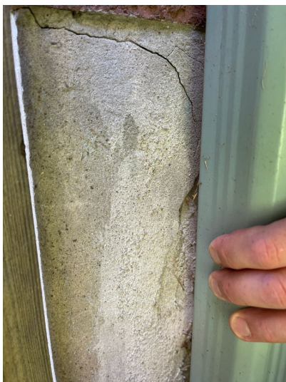
There is a corner, wedge crack behind the downspout at the left side of the home towards the rear.
