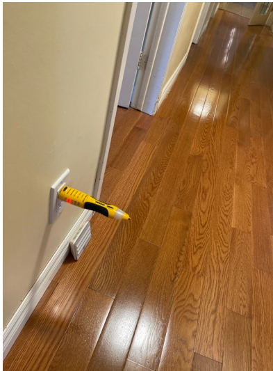
This outlet in the hallway on the main level is ungrounded. Recommend electrician repair.
