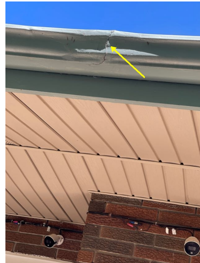
This section of gutter near the front door is damaged. Recommend splicing in a new piece or replacing the entire gutter.
