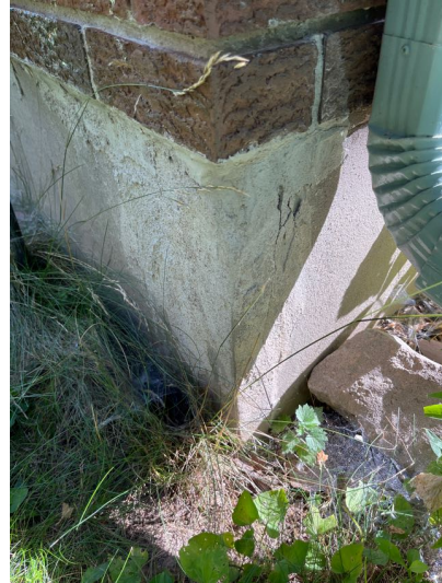
Corner wedge crack, front left corner of the home.
