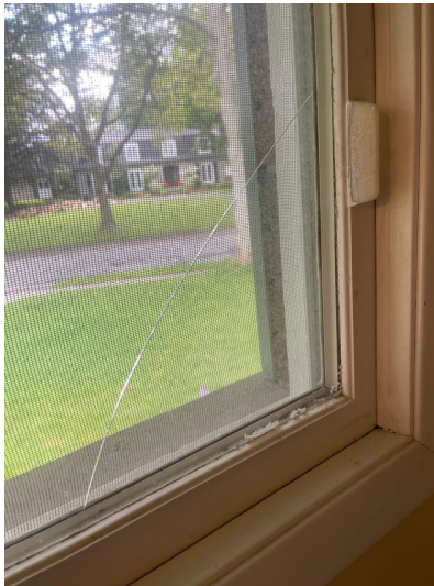
Cracked glass. Bedroom at the front left corner of the home.
