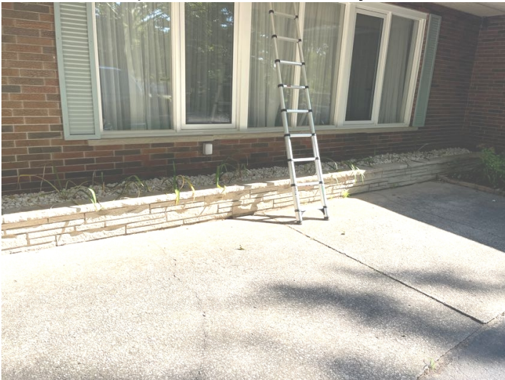
Some areas of the foundation are not visible for inspection as shown in the picture.
