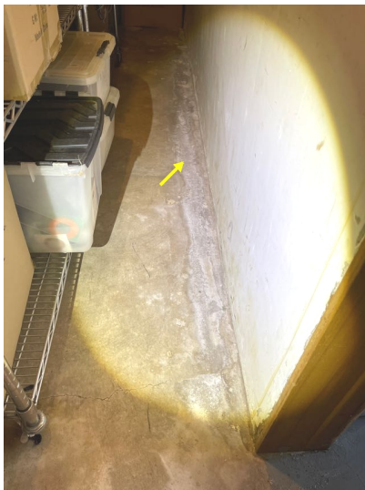
Some efflorescence on the floor in the cold room, which is located closer to the front of the home in front of the laundry room. Efflorescence indicates moisture issues. See picture F.
