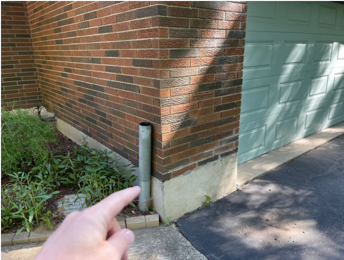
This is a unused hook up for draining the gutters underground. The gutters are now draining out onto the ground as they should be. There are a few of these abandon underground hook ups, which should be cut off and capped.
