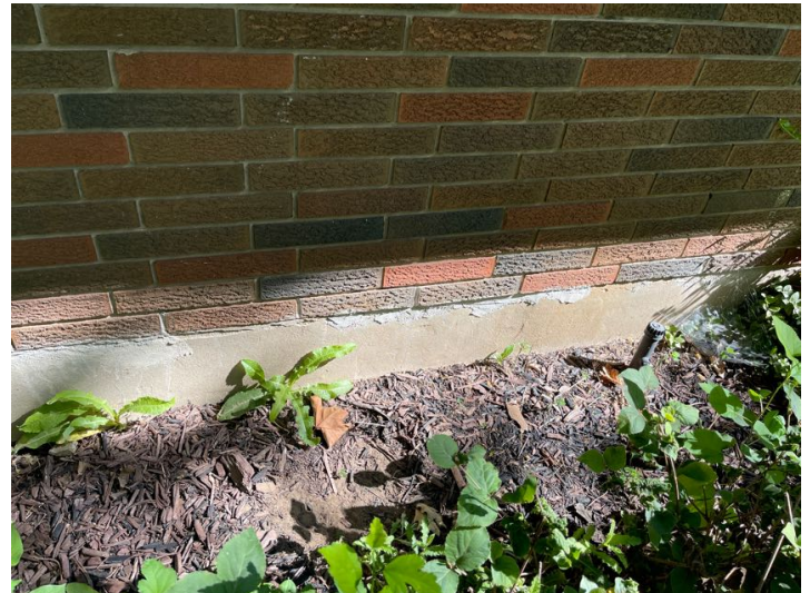
Front of home towards the left. The purging here is damaged. There is some damaged purging in several areas that has been unprofessionally patched. Recommend Mason inspect, and repair purging where needed.
